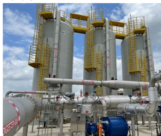
Figure 3: H 2 S Conditioning System Boilers
