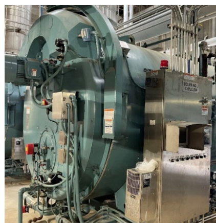
Figure 4: One of Three Steam Boilers
